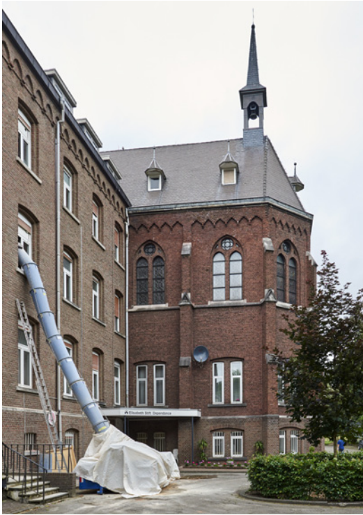
The IBA Parkstad is converting a former monastery into a home with care facilities.
